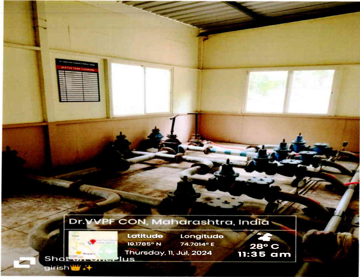
Motor pump to distribute underground
